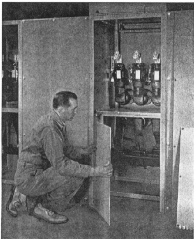
FIG. 37. Removing Barriers of Main Bus Compartment. (Busses are also accessible from breaker side of housing by removing bolted section of barrier).
